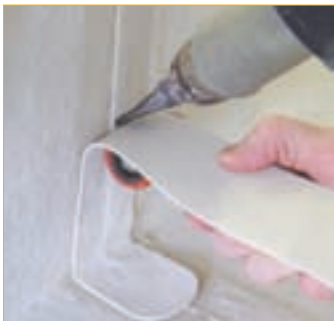
Fig 1: Waterproofing Details – Waterproofing Plus system which has built in extra protection on all critical details.
