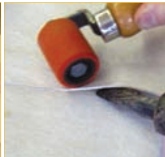
Fig 2: The Seam – Triple welded, 1 1/2" seam
